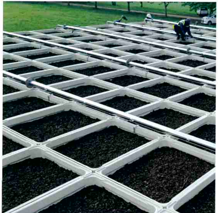
Clover Production Facility, Gauteng Treated water used for irrigation
